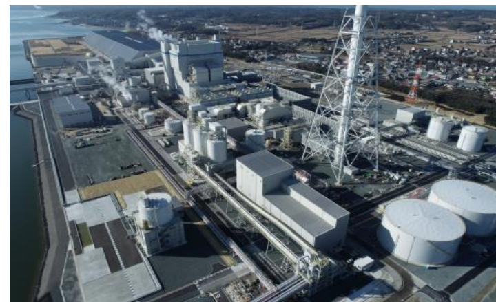
Taketoyo Thermal Power Station under construction (scheduled to start operation in August 2022)
