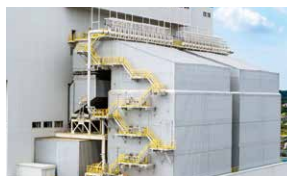
Exhaust gas denitration equipment (removal of NOx)
