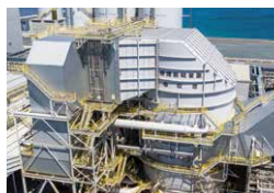
Exhaust gas desulfurizer (removal of SOx)
