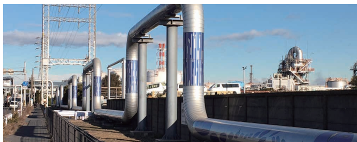
Pipe supplying steam
