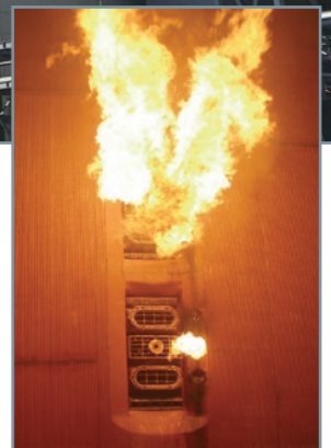
Boiler combustion status
