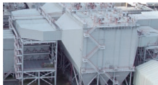
Electrostatic precipitator (removal of soot and dust)
