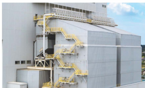
Exhaust gas denitration equipment (removal of NOx)
