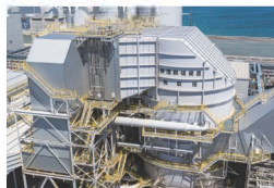
Exhaust gas desulfurizer (removal of SOx)
