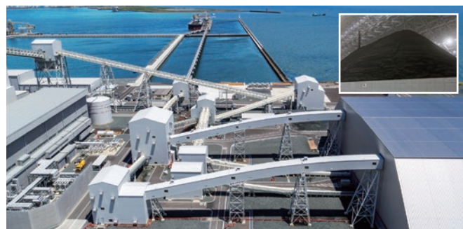
(Center) Enclosed belt conveyor (Right) Indoor coal storage yard
