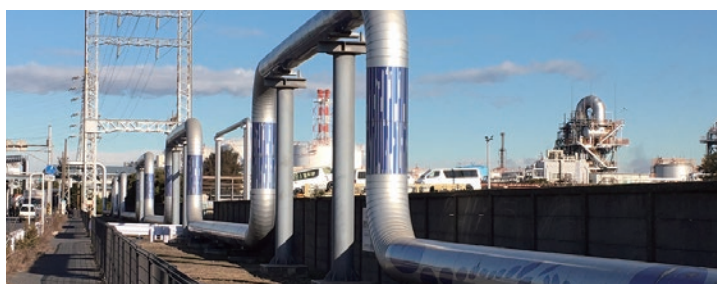
Pipe supplying steam
