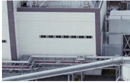
Exhaust gas denitration equipment (removal of NO x )
