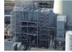
Exhaust gas desulfurizer (removal of SO x )
