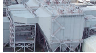
Electrostatic precipitator (removal of soot and dust)
