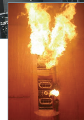
Boiler combustion status
