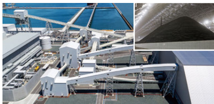
Above: Enclosed conveyor belt Top right: Indoor coal storage area
