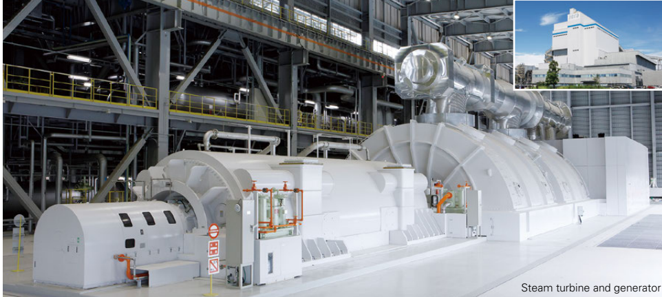
Steam turbine and generator
