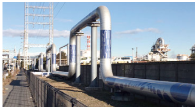
Steam supply pipe
