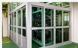
High-pressure laboratory equipment at Nippon Shokubai's Suita Research Center
