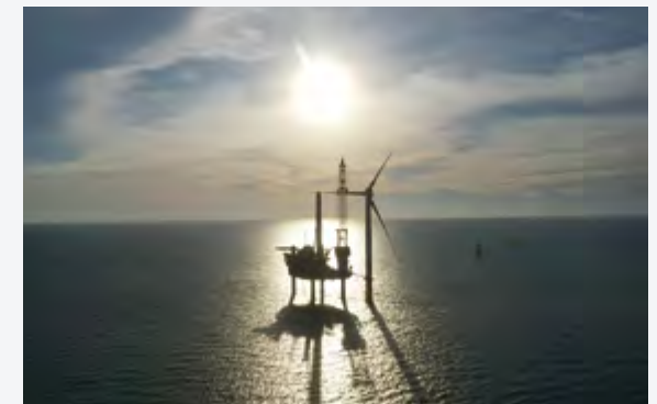
Construction of Formosa 1 Offshore Wind Farm of Power Generation Project in Taiwan © Formosa I Wind Power Co., Ltd. All rights reserved.
