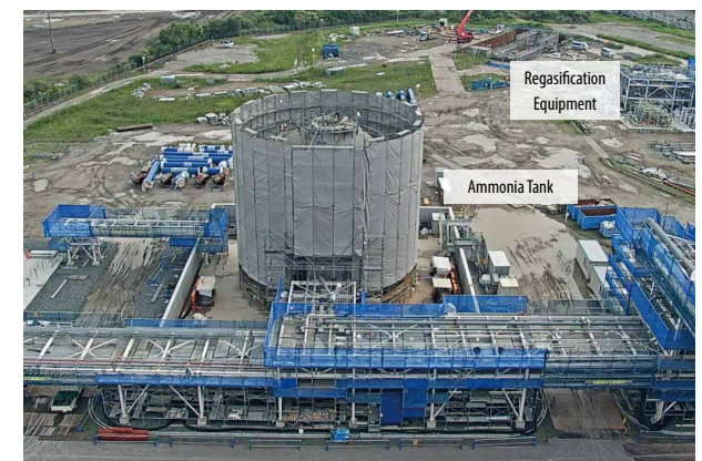
Construction Progressing on Ammonia Demonstration Test Facility at Hekinan Thermal Power Station
